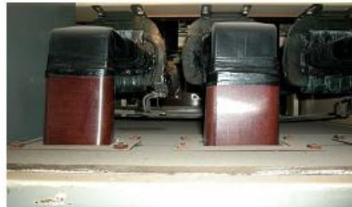
Medium Voltage Metal Clad Switchgear – Internal Bus Current Transformers
