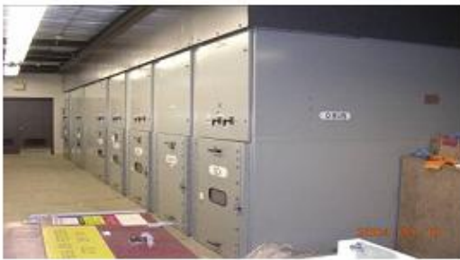
Medium Voltage Metal Clad Switchgear
