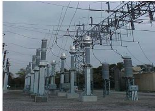
High Voltage Bus
