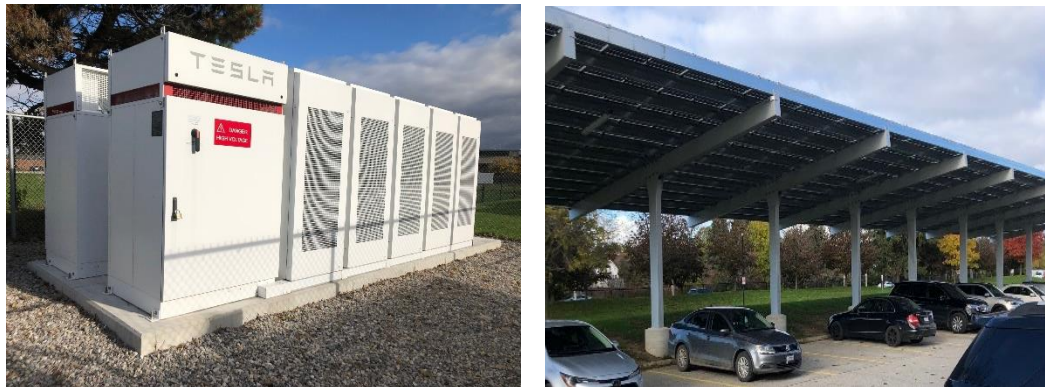
Battery (L) and solar carport (R) at John Paul II Secondary School.
