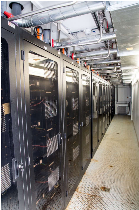
Fuel Cell Power Module (FCPM) Racks
