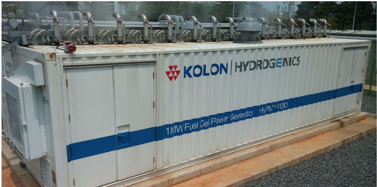
Kolon-Hydrogenics 1MW Fuel Cell Power Plant
